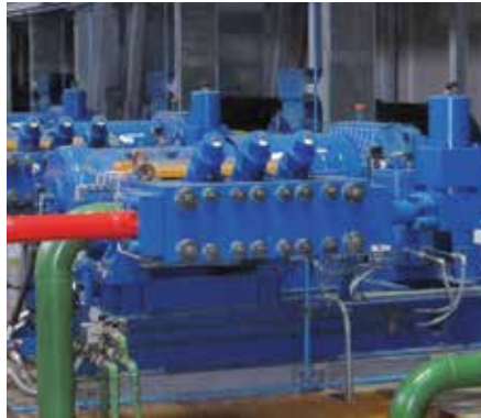
Several plunger pumps to drive an open die forging press.
