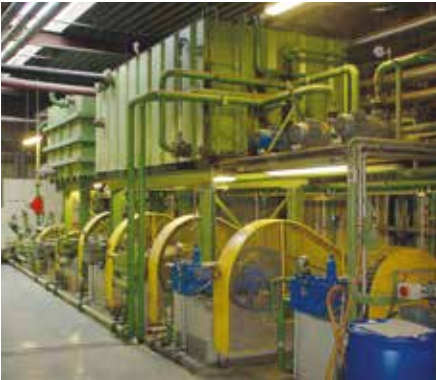
Pump units in a pressurized water system.
