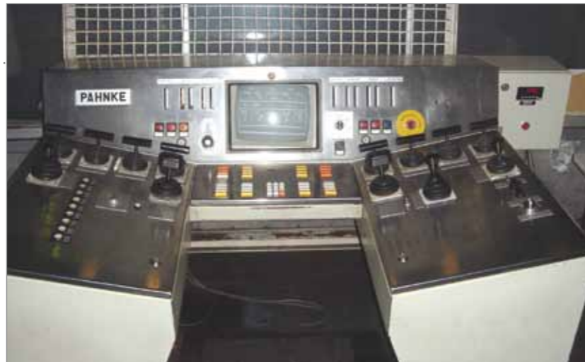
Typical PAHNKE control panel for an open die press with two integrated manipulators
