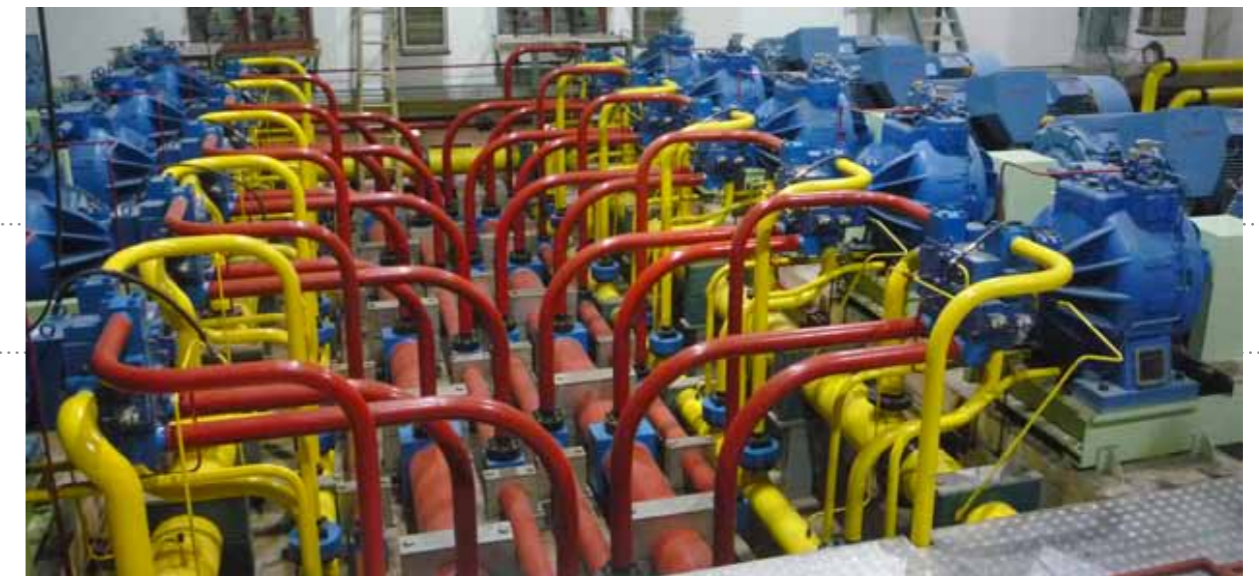
20-pump PMSD drive to the 185 MN press (RX 500)
